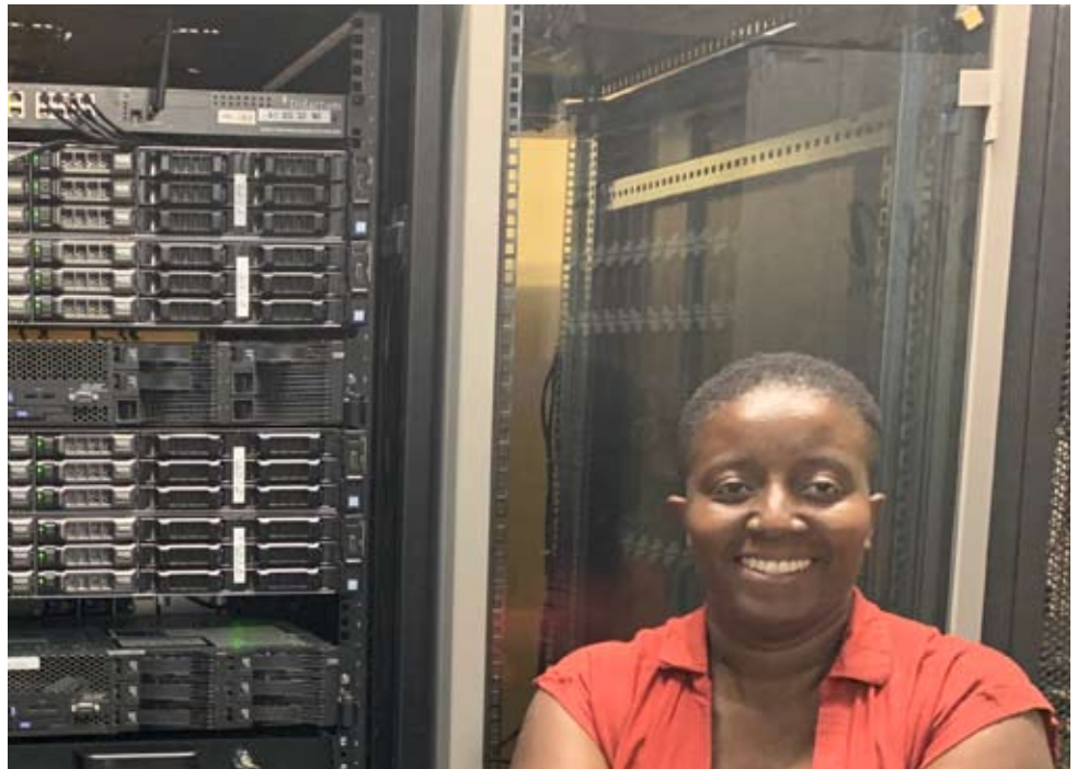
ZAMREN's server room
