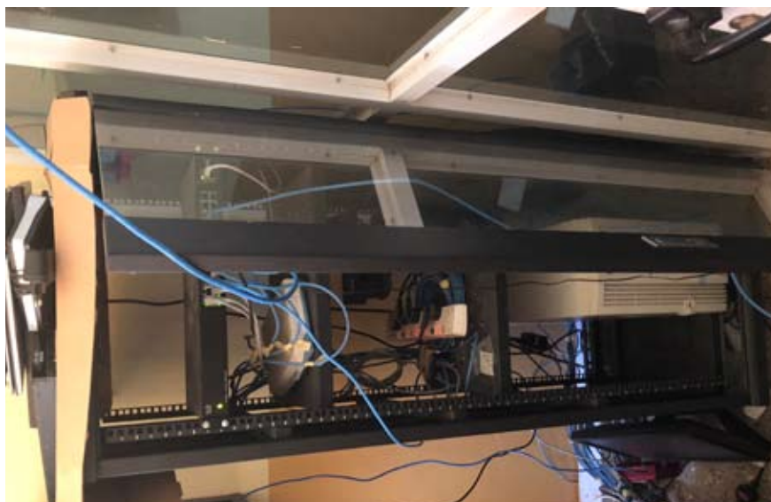
A view of SARI’s “server room”, during Hixson’s first visit to Nyankpala, Ghana in October 2018. At that time, SARI lacked adequate bandwidth for their researchers and their server equipment was located in a corner of the IT manager’s office which lacked constant climate control, was open to non-IT staff access, and had a number of wiring problems.
